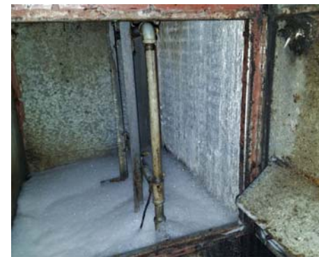
Figure 3: HRU washdown section showing clean coil.
